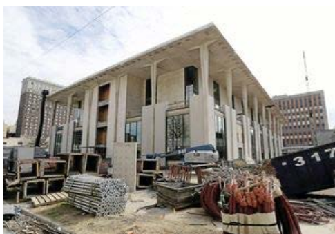
Construction continues at Tulsa's Central Library on Friday. The library is expected to reopen this summer. CORY YOUNG/Tulsa World
