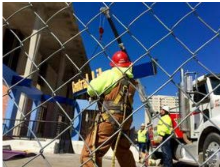
Workers take down the last sign at downtown Tulsa's Central Library. The branch is undergoing a $50 million renovation. Credit Matt Trotter / KWGS
