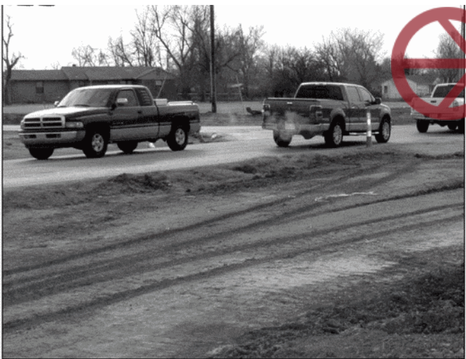
HAYLIE SMART/OWASSO REPORTER Construction crews are in the process of widening the intersection at North Garnett Road and East 106th Street North. The city of Owasso anticipates completion of the intersection in April. Crews will widen the intersection to five lanes for both roads.
